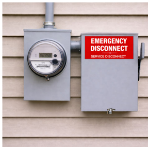
National Electrical Code 225.41
